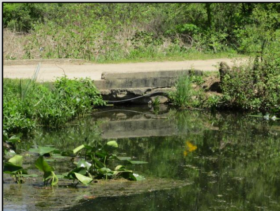
Outlet on North End
